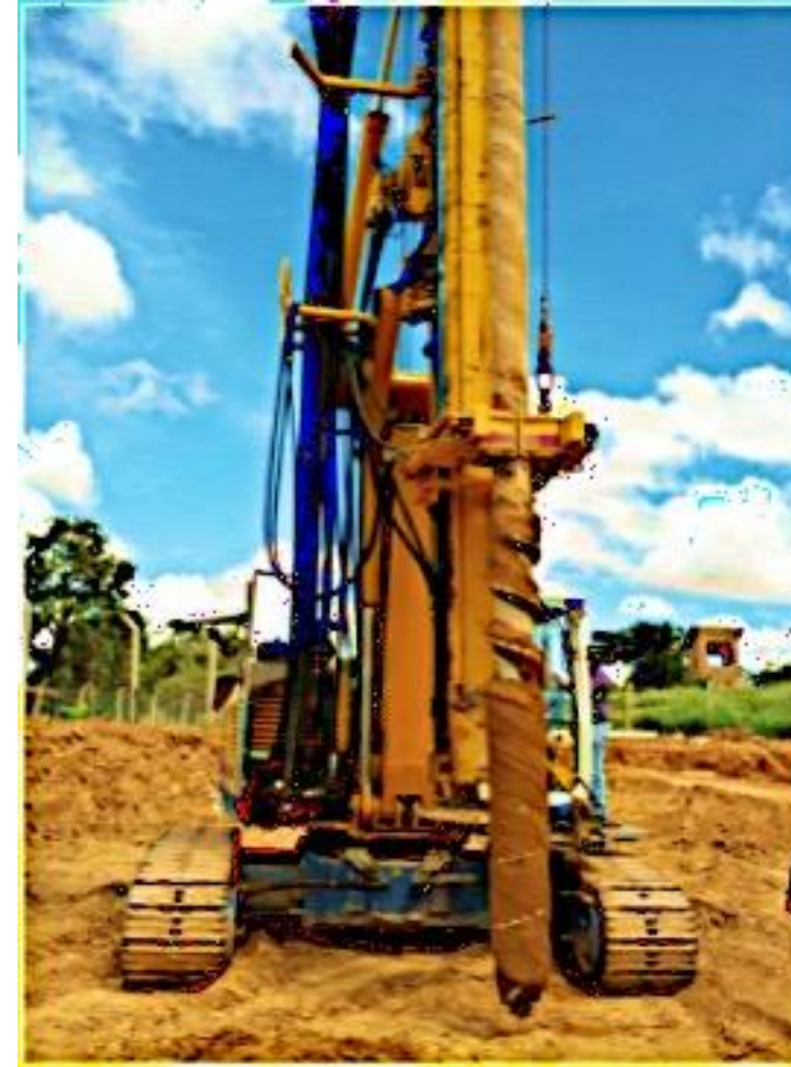
Full displacement auger pile (FDP) with EB achieves high shaft and toe resistances.
