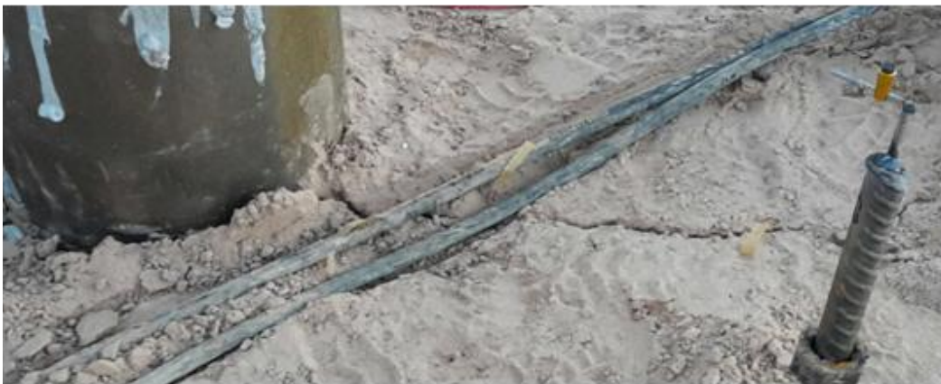
Fig. 16b Photographs of cracks in ground surface stretching from one pile toward the next along the side of the group.
